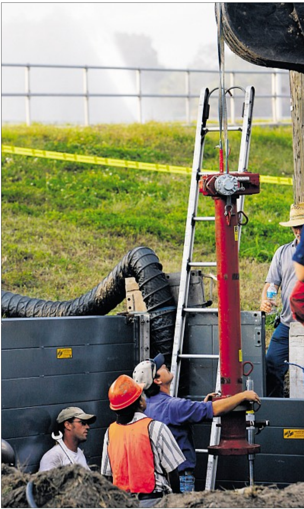
As water cannons spray close by, Mike Clark of Houston lines up a gate Tuesday to help stop an ammonia leak near the Alafia River. The breach created transportation nightmares. Story, 3B
